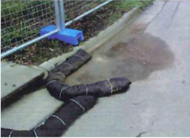
Gravel sausages require de-silting when sediment has built up to 1/3 the height of the measure, when the built up sediment is preventing the log from working effectively, or when the sausage is clogged and run-off can no longer flow through it.
